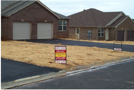
Straw mulch can be used to both prevent erosion and minimize dust from a site. Photo credit: Barry Tanning, Tetra Tech.
