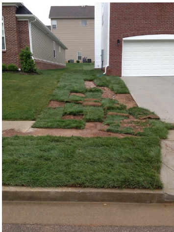
Sod installation failure. Sod needed staples. Photo credit: Barry Tanning, Tetra Tech
