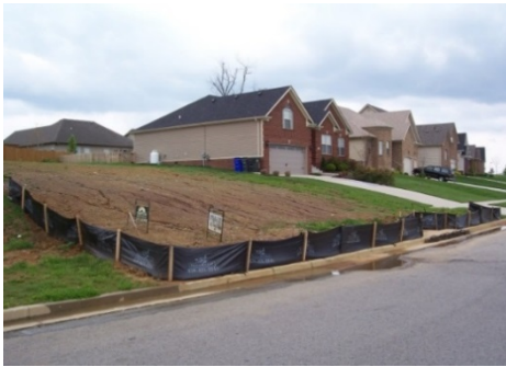
Site with properly installed silt fence. Note that fence posts are installed on the downhill side of the fabric. Photo credit: Barry Toning, Tetra Tech
