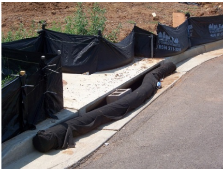
Typical filter bag inlet protection installation. Photo credit: Barry Tinning, Tetra Tech
