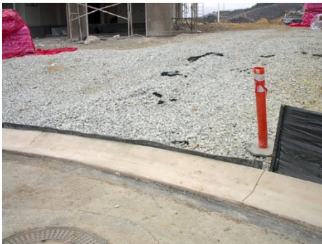
Good application of rock exit pad. Note short section of material against curb that is keeping rock from leaving site. Photo credit: John Kosco, Tetra Tech.
