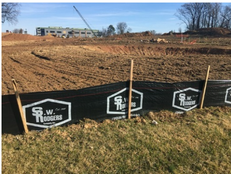
Ensure silt fence is dug into ground to prevent runoff from escaping underneath. Photo credit: John Kosco, Tetra Tech
