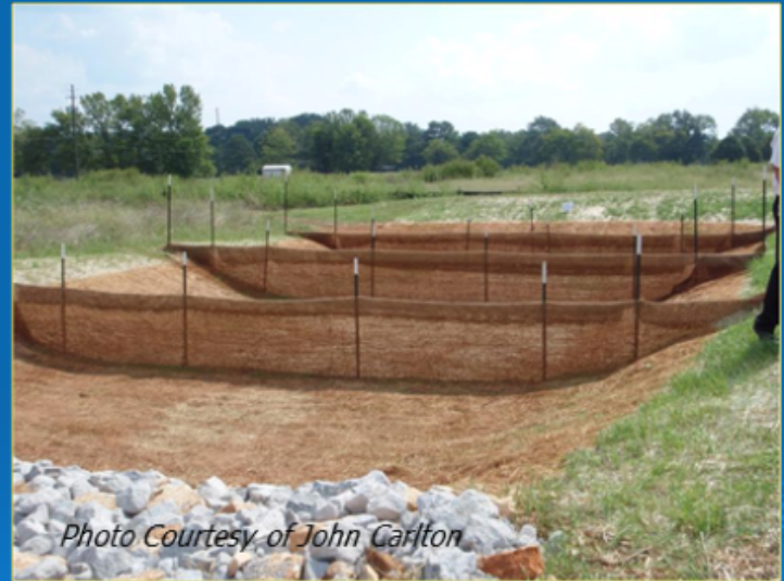
Good Staged Basin Vegetated Slope
