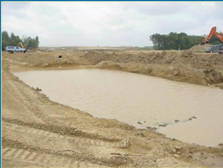
Bad Large Single Basin Slopes Exposed
