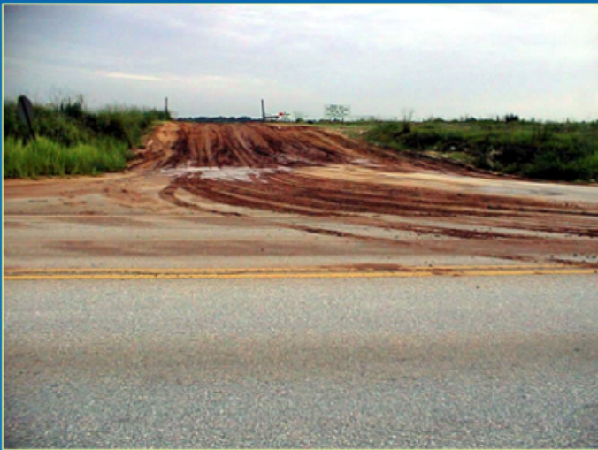
Bad Tracking of Soil onto Roadway
